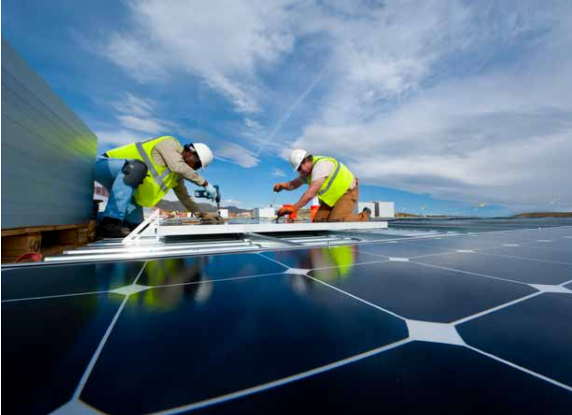
Namaste Solar workers Wes Van Norton (left) and Scott Pieper (right) installing rooftop solar panels on a parking structure.
